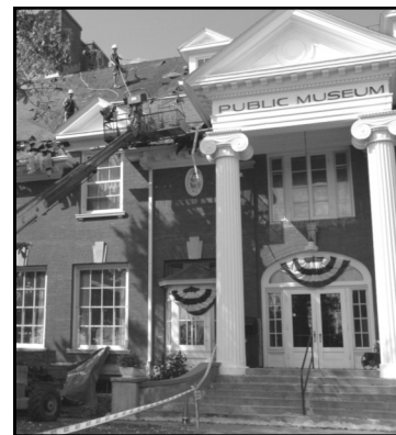
Our new roof was completed this fall. You can still make donations to this project.
