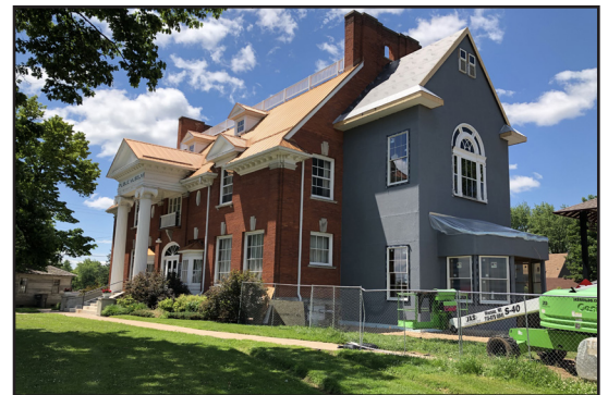
During this past winter we fundraised, planned, and waited for spring. By the end of June, the addition was taking shape. (original façade on top, addition taking shape below) Once completed, work on the interior will begin in earnest.
